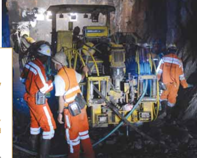
The Yalea underground mine development made a record advance of 605 metres in March
