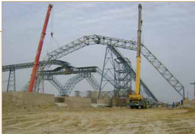
Erecting the conveyor arch support over the new ore stockpile at Loulo.
